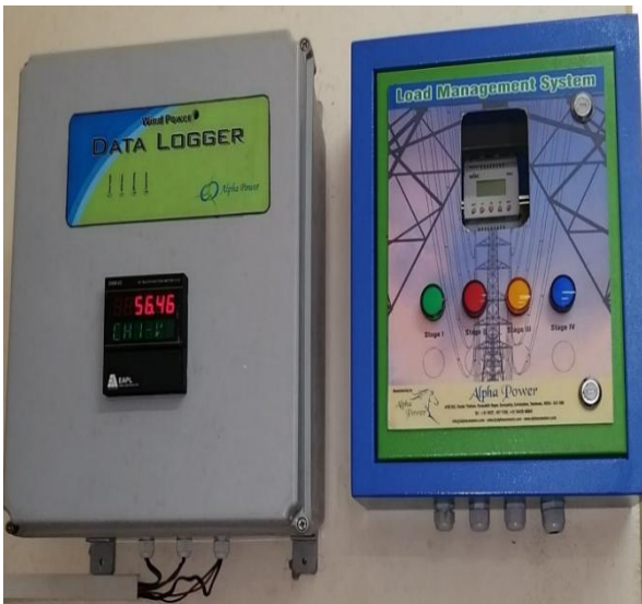
Figure 4 Data logger and Load Management System
