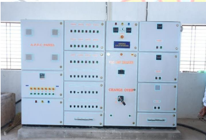
Figure 6(b): Electrical Control Panel
