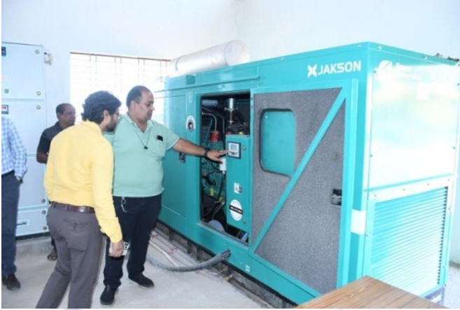
Figure 6(a): Electrical Control Room
