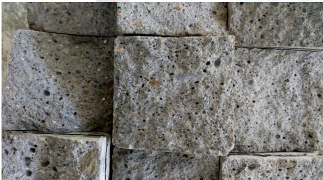
Fig.7:Voids Present in Mortar Sample
