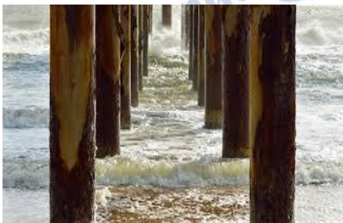
Figure. 1 deterioration of concrete due to aggressive conditions
