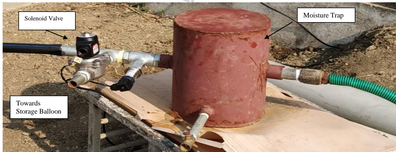
Fig. 6 Proposed system installed at Sanjeevan Oldage Home
