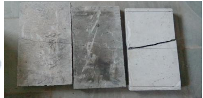
Figure No. 6 – Cracking of panels
