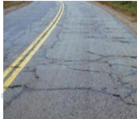
Fig: block cracking
