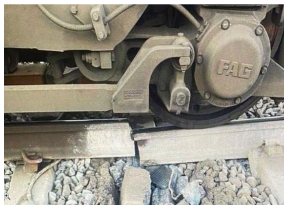
Fig. 1 Part of the track which was completely broken Ultrasonic is used for the surveying process also, other important element is This system used during road track examination. System is suitable to descry deeper cracks
