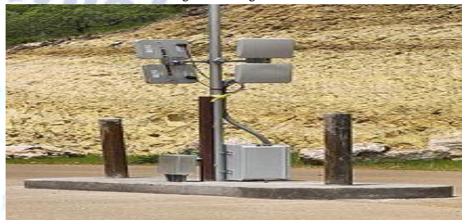
Figure: 4. An RFID system in use for traffic monitoring
